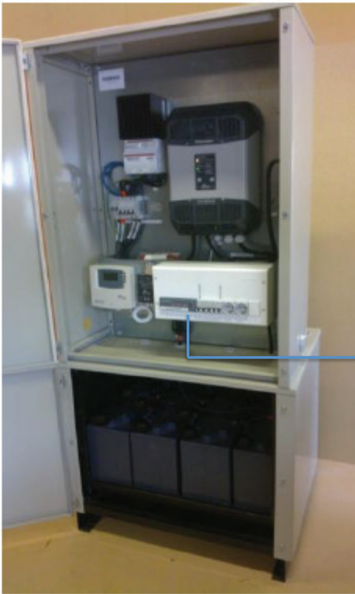
Off grid electrical cabinet Control, manage, store energy
